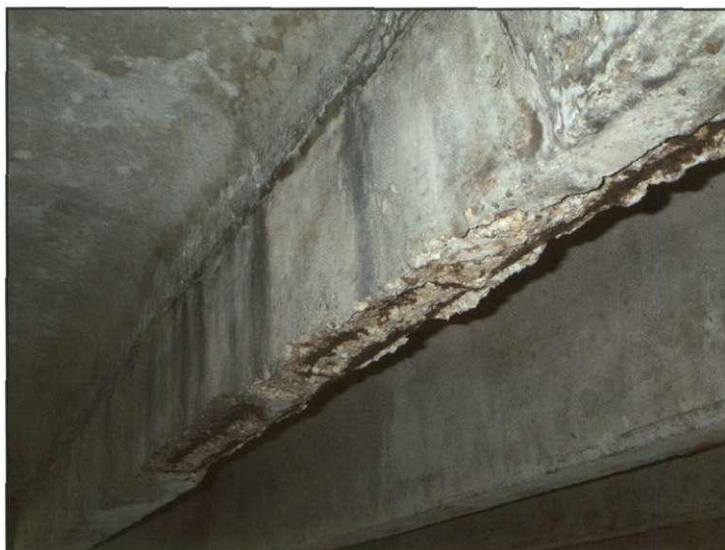
Figure A1 Spalling of concrete on downstand beams.
