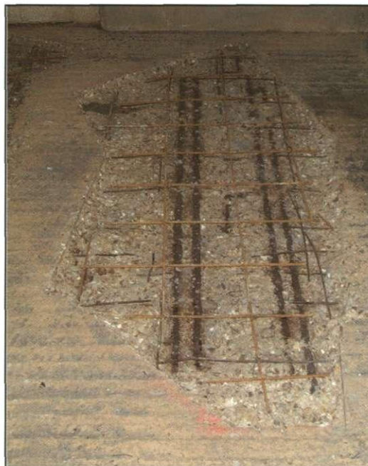
Figure A2 Area of spalling on the deck.
