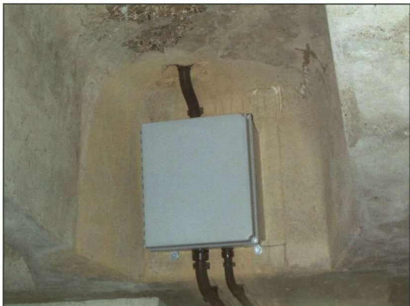
Figure A5 Typical termination box.
